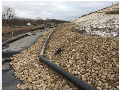
Toe of slope horizontal gas collection
