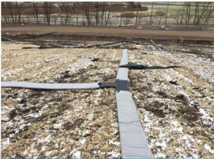
Gas collection installed below geomembrane cover
