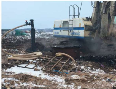
2. Vacuum box installed and connected to collection system
